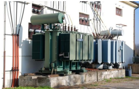
Figure 2. A 35/10 kV substation in the Brčko District of Bosnia and Herzegovina (source: https://radiobrcko.ba/vijesti-brcko/u-toku-redovan-godisnji-remont-cvornih-trafo-stanica-u-distriktu/ ).
