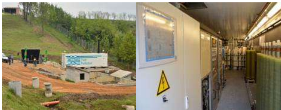
Image 1. Purification of landfill filtrate at the Ramici landfill Source: Author's image
